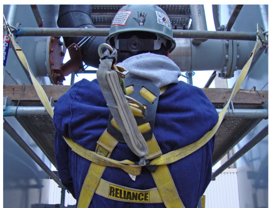
Incorrect Use of Shock Absorbing Lanyard as a Positioning Device
